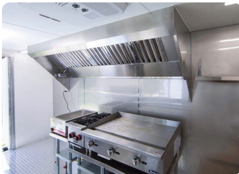
Commercial Kitchen Hood
